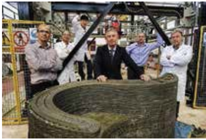
Figure 3. Freeform Construction team at Loughborough University displays a composite wall prototype. Photo: Dr. Richard Buswell and Professor Simon Austin, Loughborough University.
